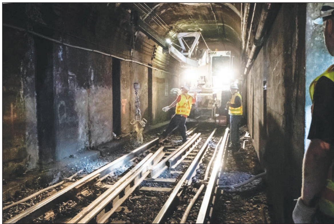
The MBTA will close the Blue Line from Government Center to the Airport for nearly two weeks next month for tunnel repair work.
